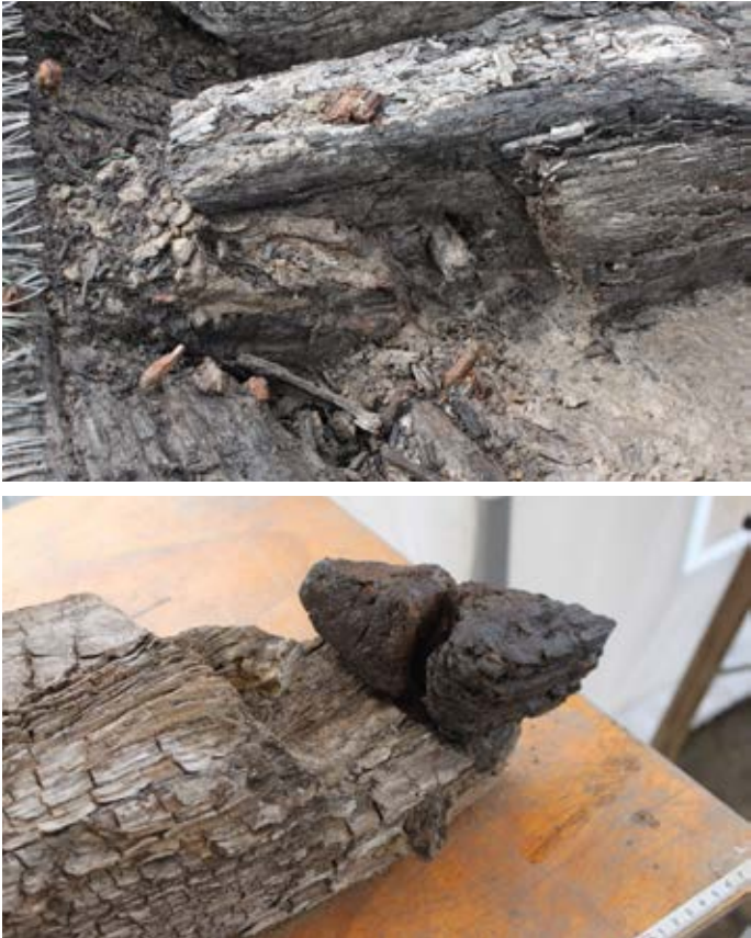
Fig. 32. Connection of floors timber to futtock by two horizontal treenails and a rebate in the floor (photo IFMAF).
